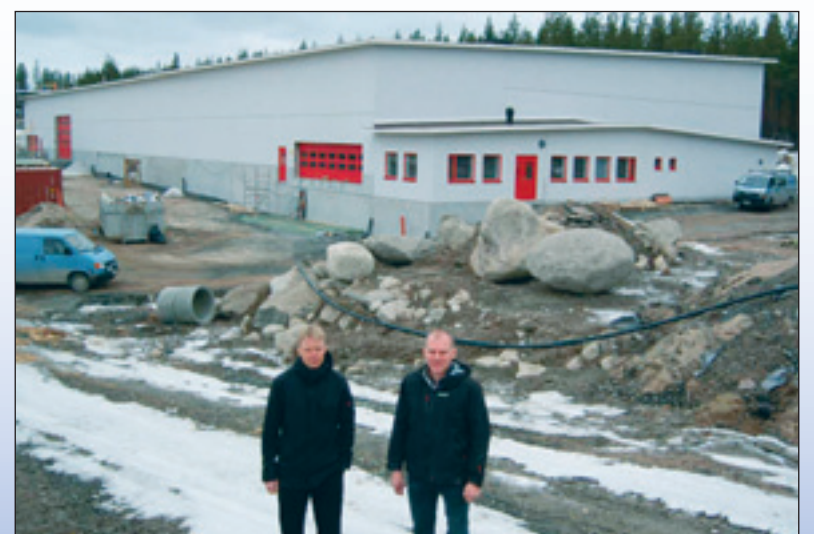
Mr. Kurikka and Mr. Hietikko are very satisfied that the new factory project finishes in timetable.
